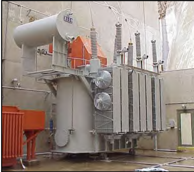
Figure 1 – Typical GSU Three-Phase Transformer.
