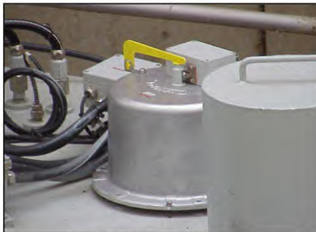
Figure 30 – Photograph of a Pressure Relief Device.
